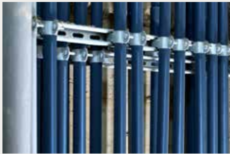
Tap water piping for architecture and column piping
