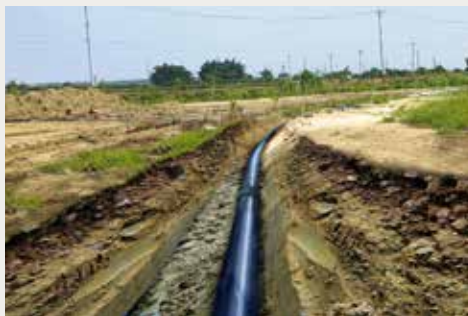
Sprinkle and irrigation piping
