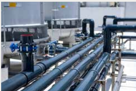
Chilled water piping
