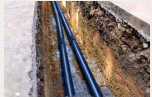
Water pipe and electrical conduit used for seismic zone or high-pressure area (road)
