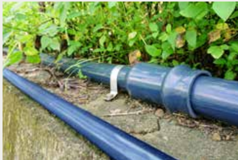
Tap water piping in mountain area
