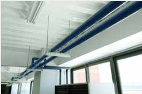
Transportation of chilled water for air conditioning system
