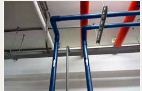
Dynamic flow sewage piping
