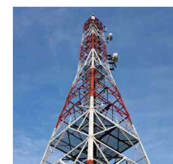
5G Base station
