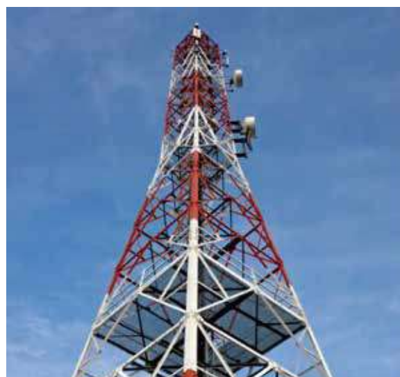
5G Base station
